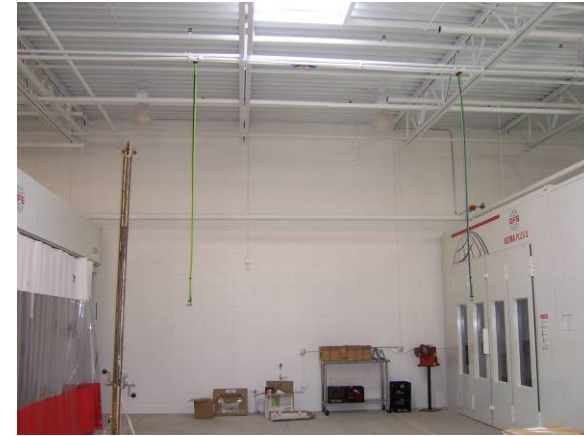
Hose and Pipe Drops
